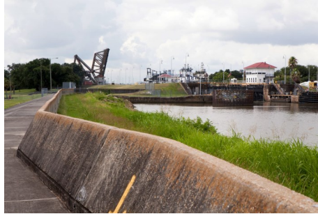
Stock photo of the Wagon seller levee prior to the collapse
